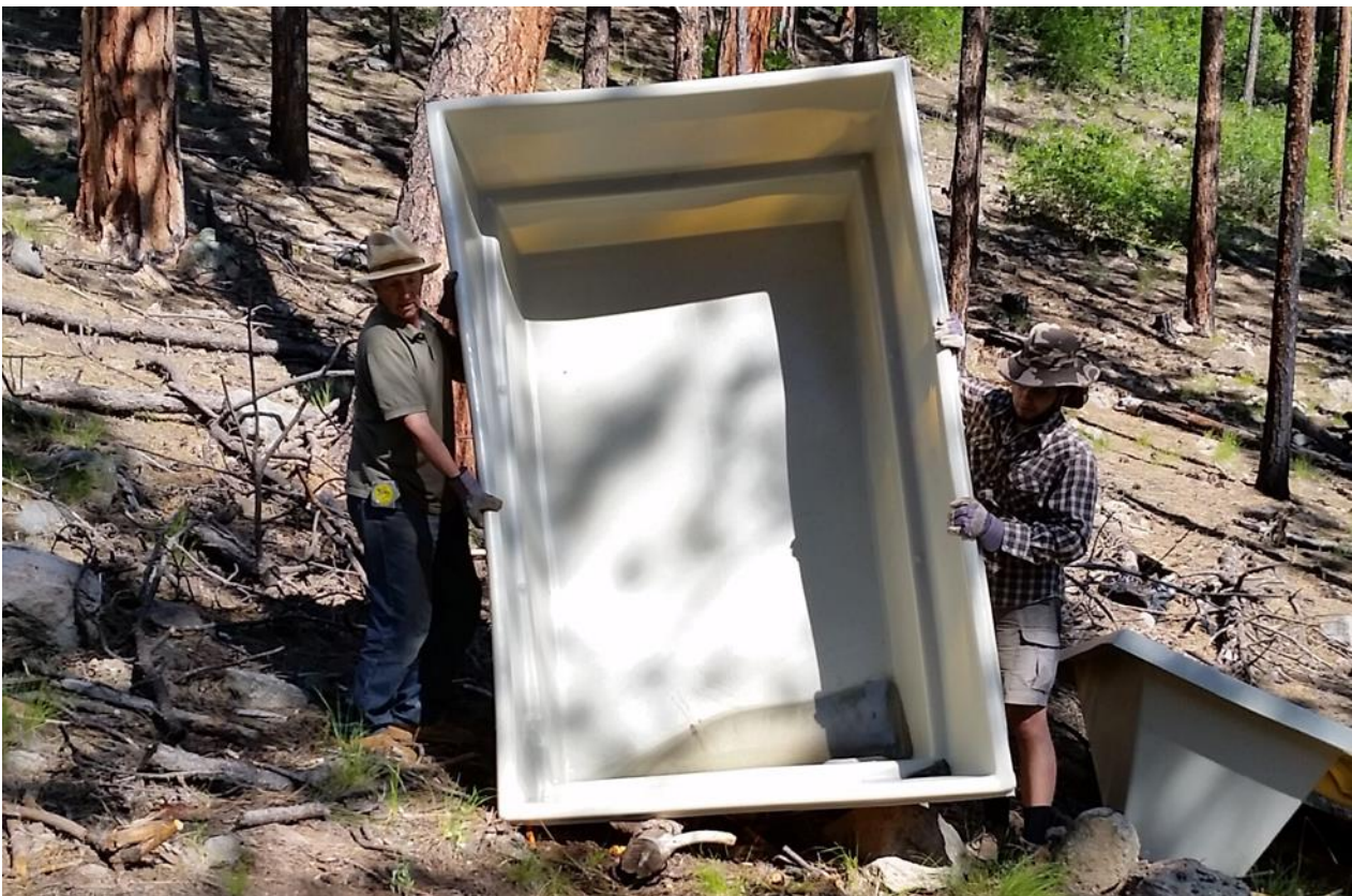
Getting ready to place the tank in the hole close to the cabin.
