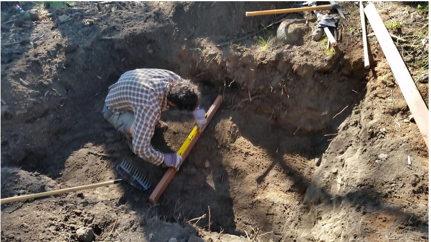
Hole for the tank at the cabin being made, making sure that the base for the tank is even all throughout.
