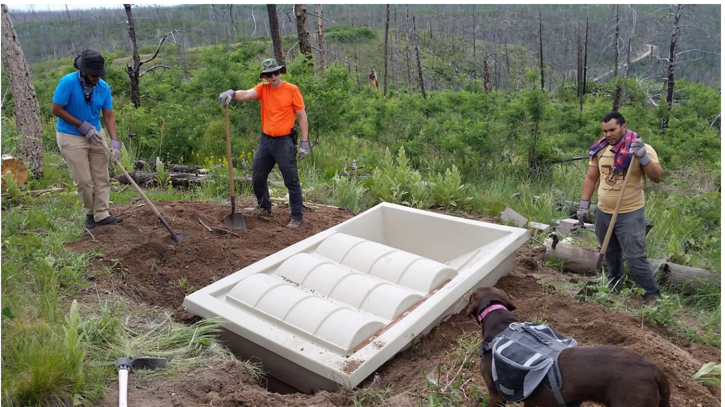
Filling the sides of the tank with dirt and rocks to give it stability at the ranch.
