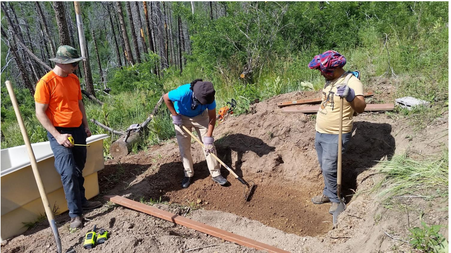
Hole for the tank at the ranch being made, making sure that the base for the tank is even all throughout.
