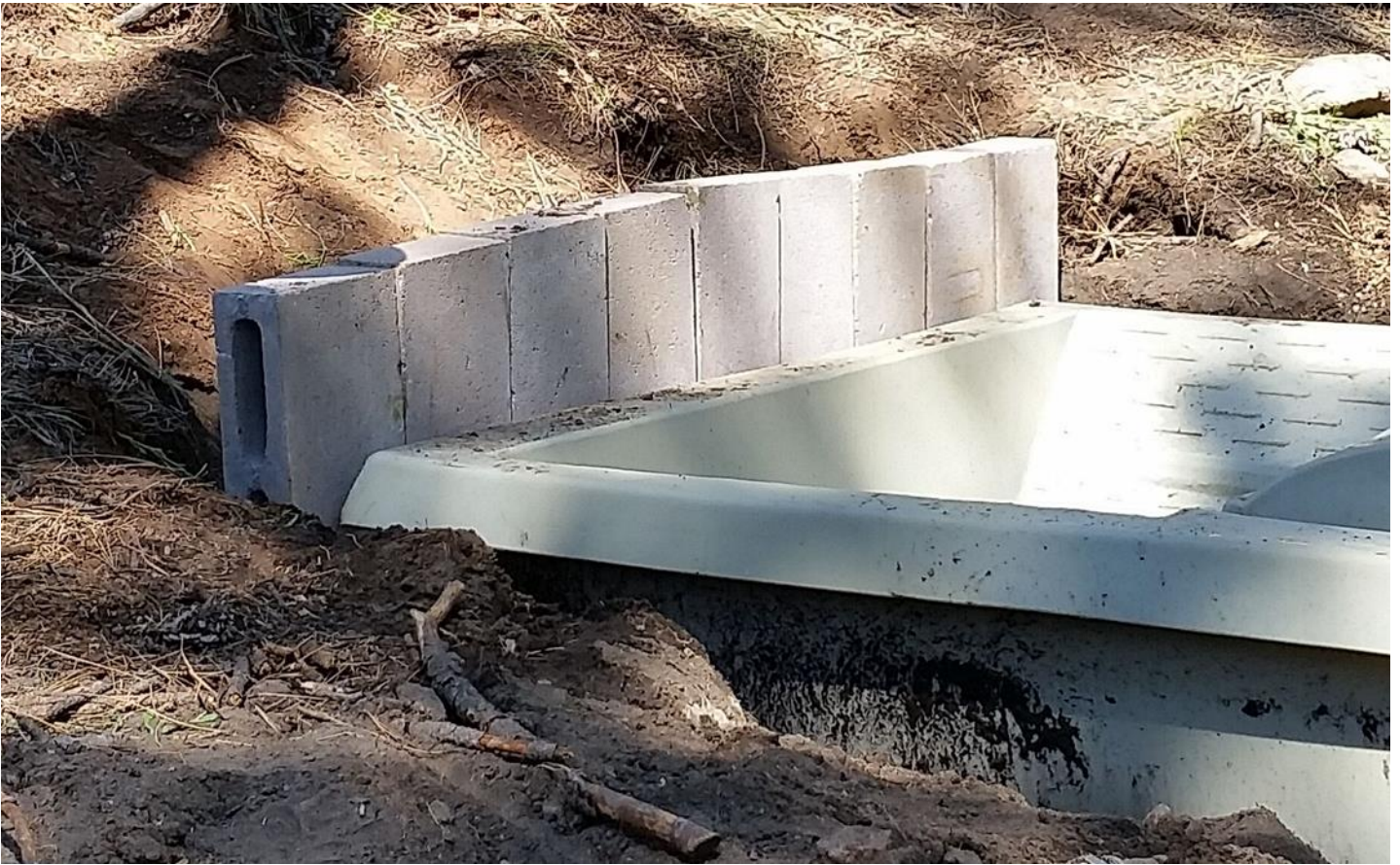
Placement of a brick wall in the water drinking side of the tank as to prevent debris from falling in.
