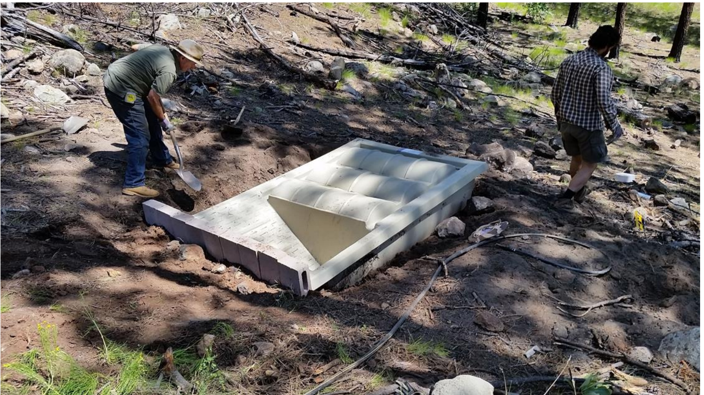
Filling the sides of the tank with dirt and rocks to give it stability at the cabin.
