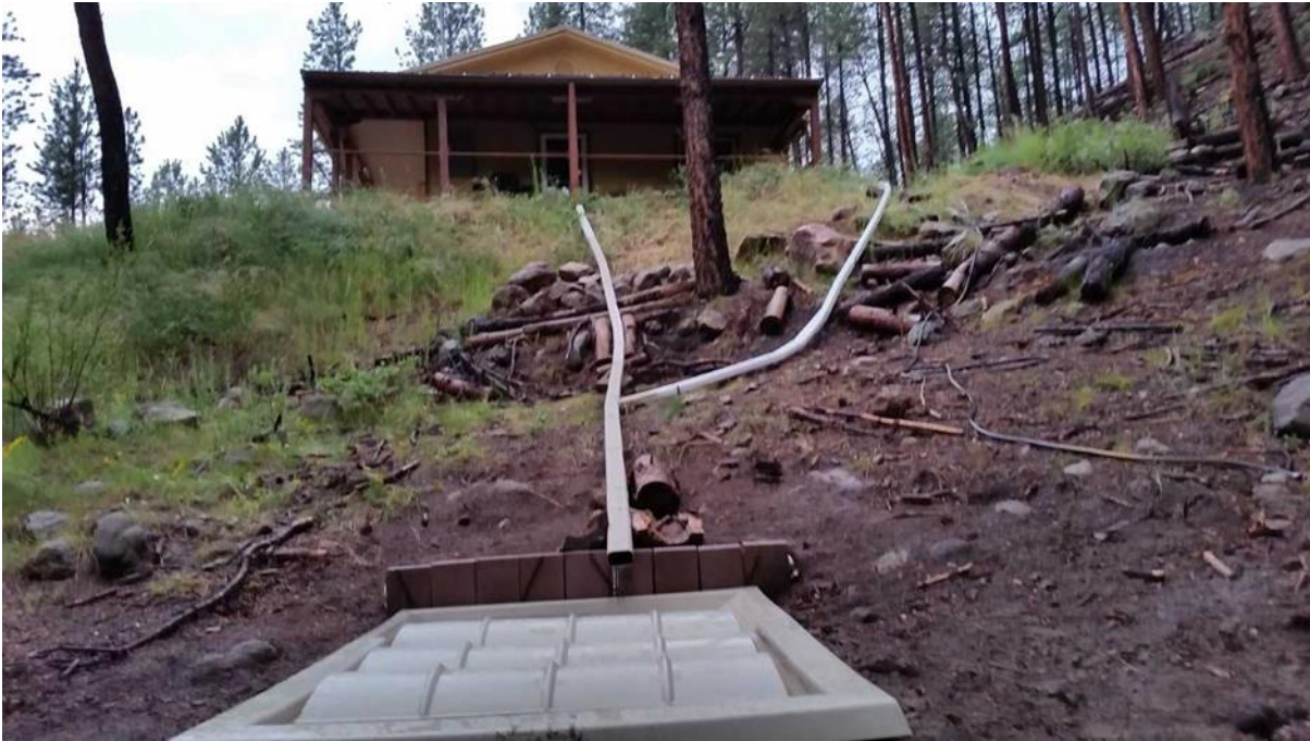
Connection between the water collector and the tank at the cabin.
